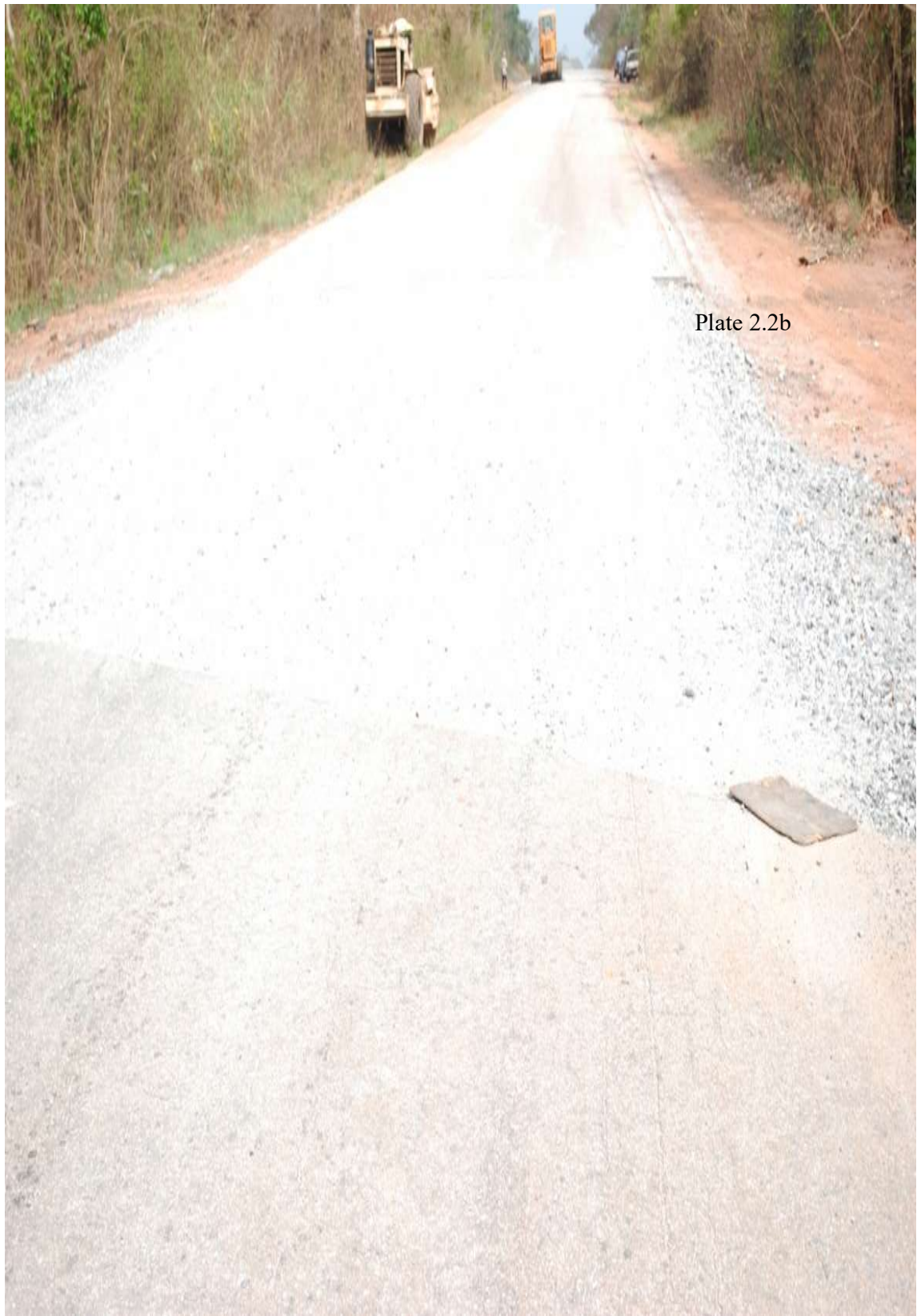
Plates 2.2a and 2.2b: Failed Section at Location 1
