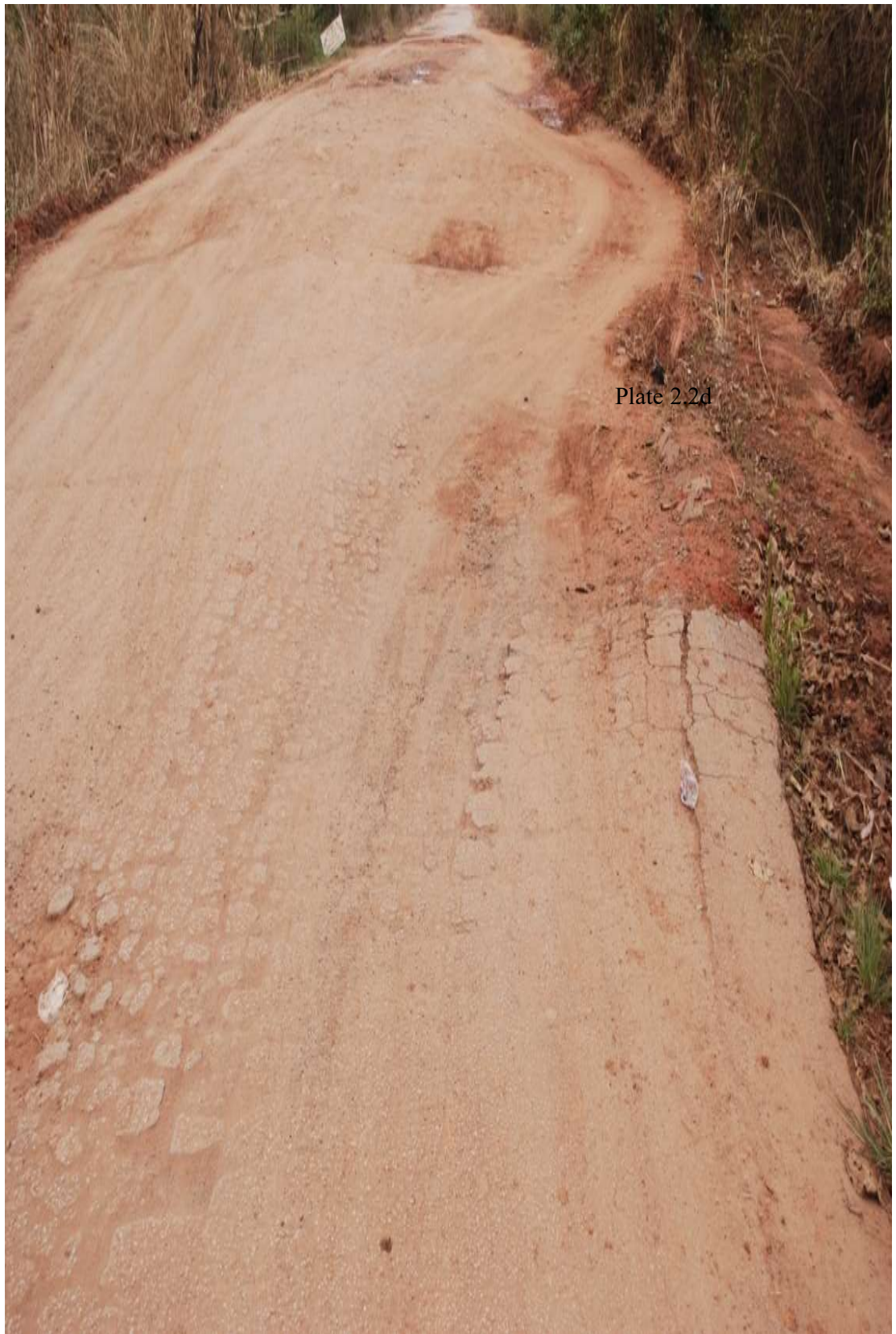
Plates 2.2c and 2.2d: Failed Section at Location 2
