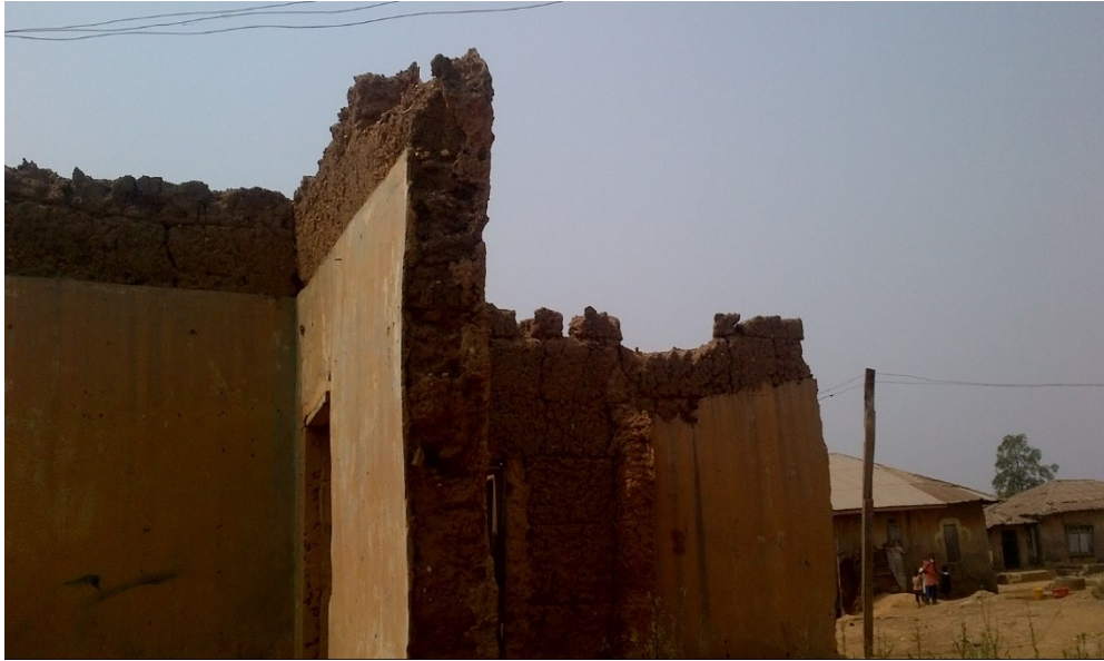
Plate 4.7: Devastated building and a standalone tree at Morgana Compound, Idiarere, Ibadan
