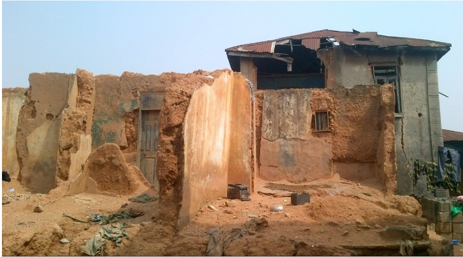
Plate 4.5: Devastated and non-reinforced high rise building at Buildings at Idi-Arere Ibadan
