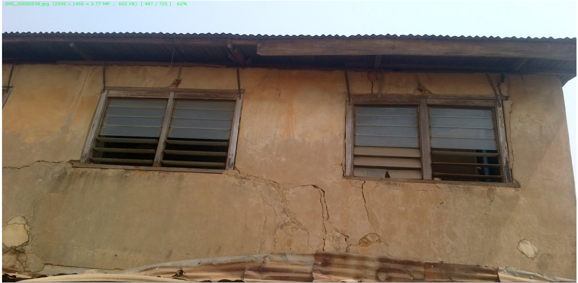
Plate 4.12: Anchor /Tight Belt Nailed to Window Frame and Openings at Isale Bode, Ibadan
