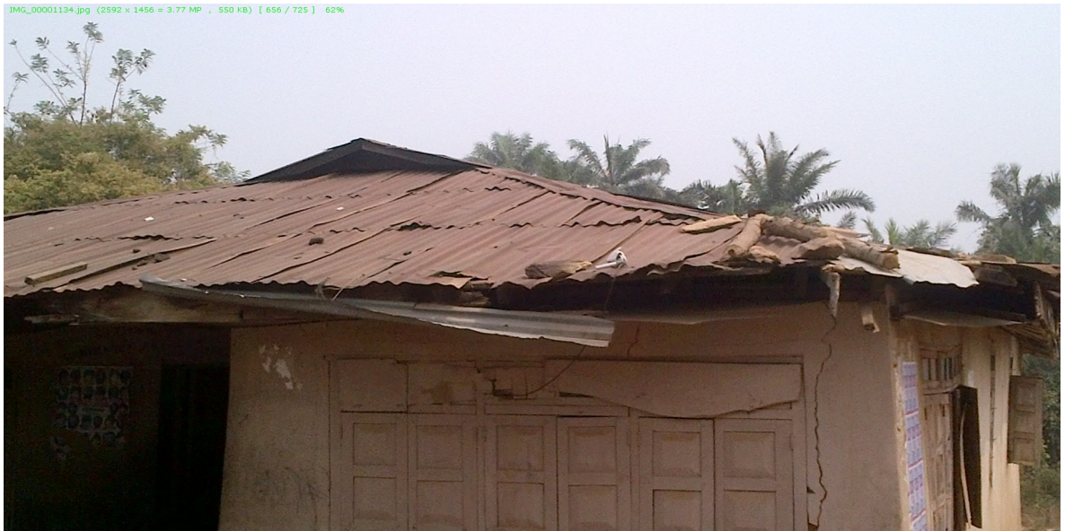
Plate 4.13: Heavy Material Placed on the Roof to Prevent Roof from Windstorm Damage in Idi-Ayunre
