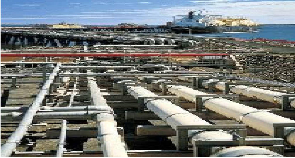
Figure 2.3: LNG Delivery Facility with Tanker, United State Source: NGSA
